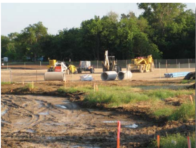
Bill Schweitzer took these pictures of the progress on the natural gas pad site next to the club
